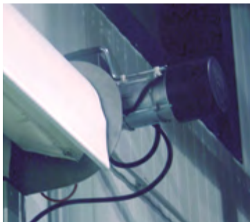
Detail of motor
